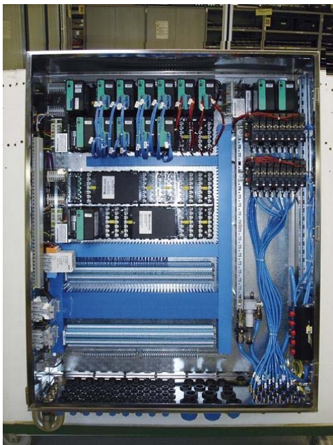
Fig. 2: Remote I/O acting as an intelligent junction box
